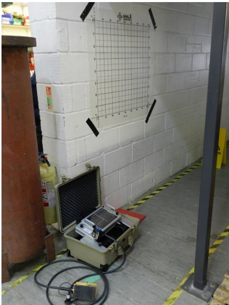
CX12 being used to identify any cavities behind a breeze block wall.
